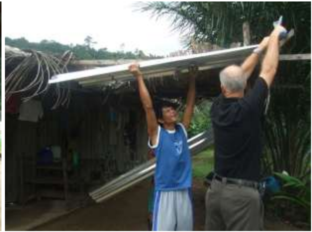
Lack of a ladder meant the tallest person had to hammer
